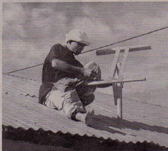
One of the Lao company's engineers installs the base of a solar panel in recently ravaged Nias, Indonesia.
