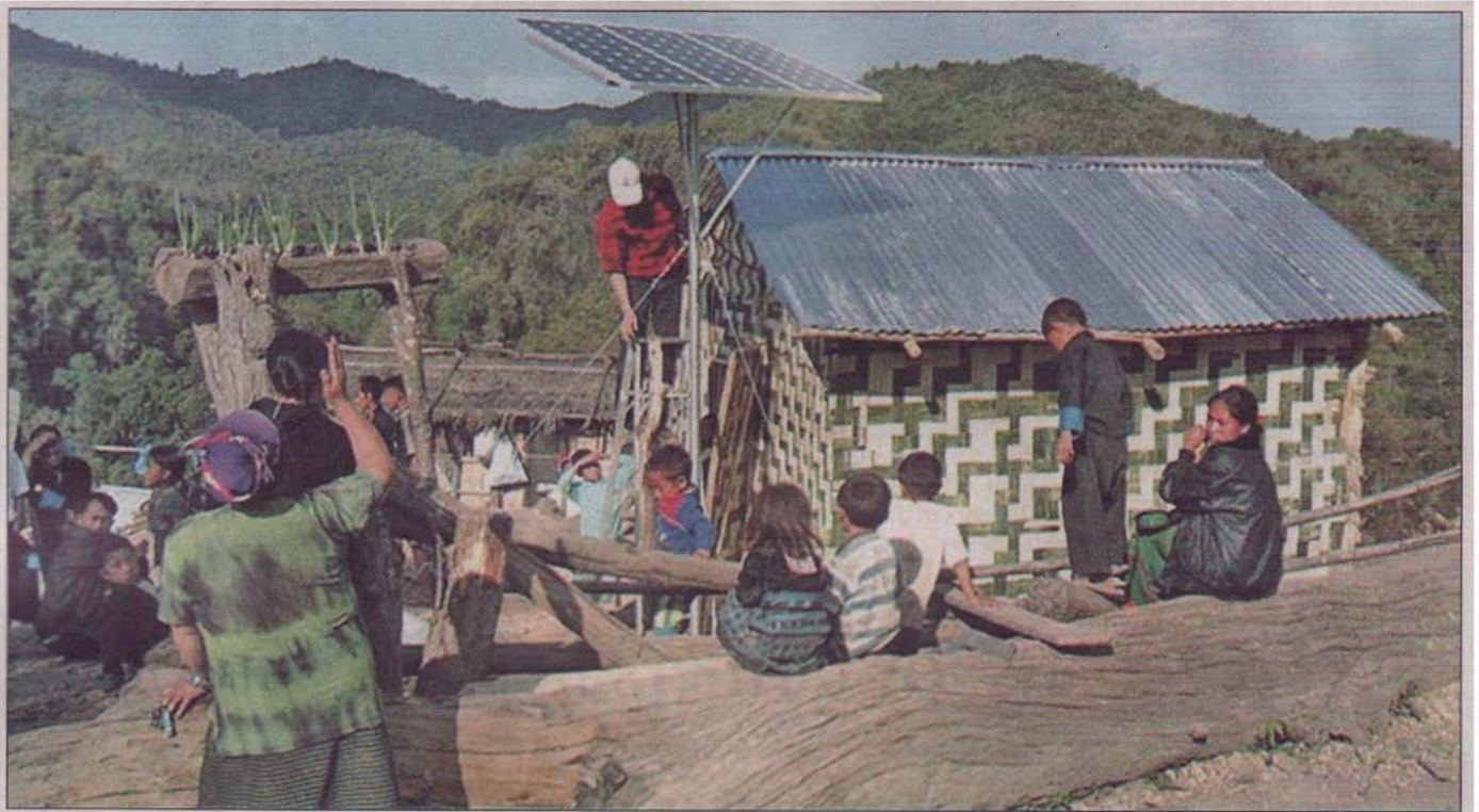
Sunlabob provides efficient solar panels to bring energy to rural families.
